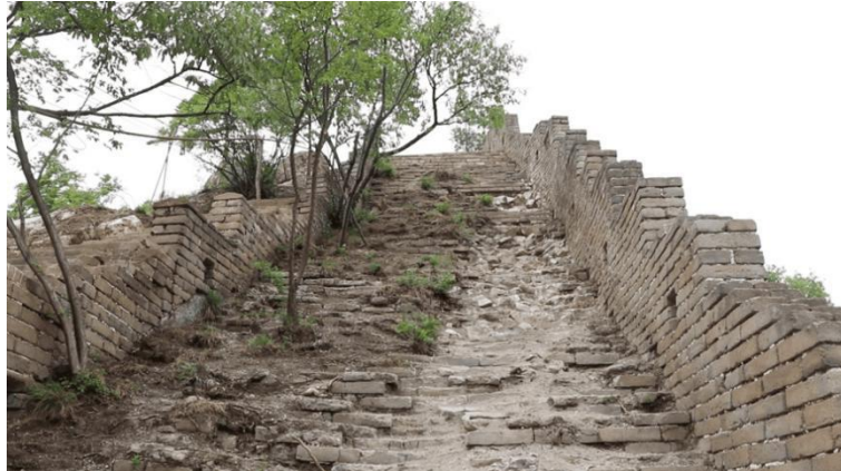
Figure 5: Jiankou Great Wall before restoration (photo source: the official website of the China Foundation for Cultural Relics Conservation).
